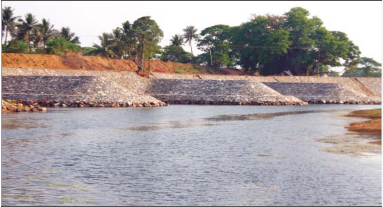
Kusabhadra Left Embankment (Slope protection work and spur at Behera completed under RIDF)
