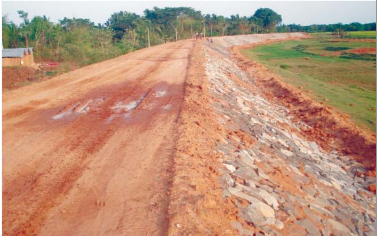
Old Maratha Embankment (Rising and Strengthening of embankment & Slope protection work completed under RIDF)
