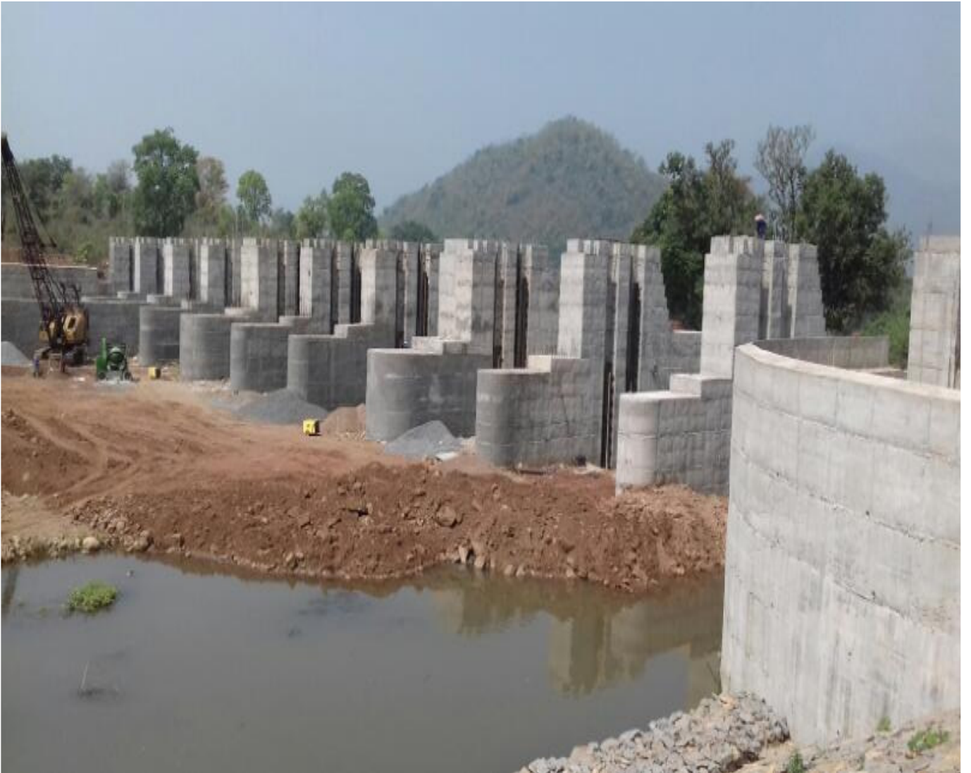
Mahendratanya Barrage across river Mahendratanya at village Dambapur (Rayagada Block of Gajapati District)
